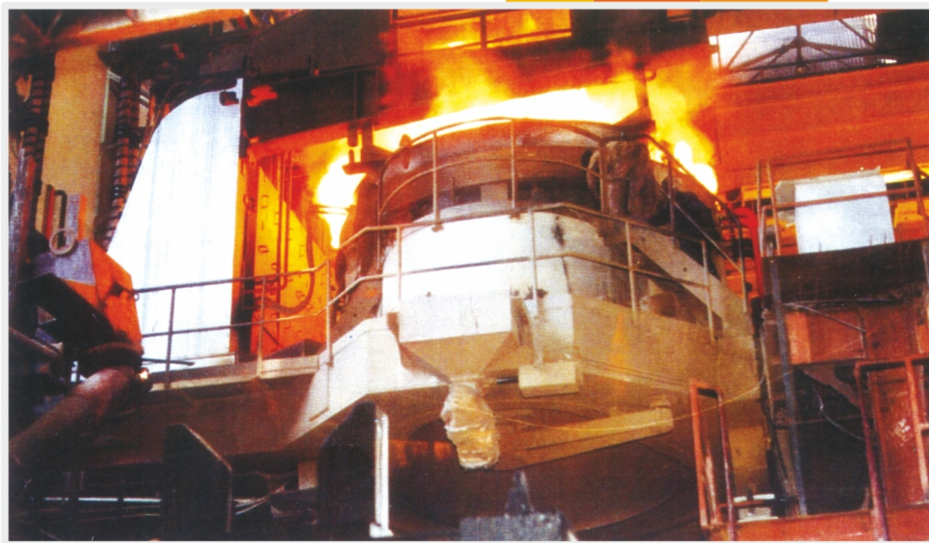
45 Tonne, UHP 36 MVA Arc Furnace type AL-460
